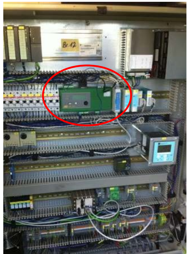
Control cabinet at well no. 17 with OTT netDL1000 and bus converter for Profinet connection to SPS
