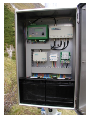
Technology at the measurement station
