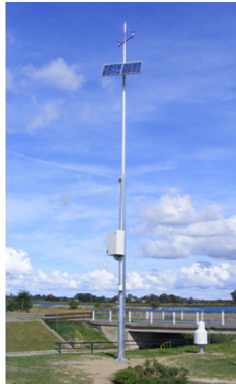
Measuring station on a 10 m mast with solar panel
