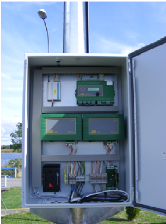
Steel cabinet with OTT LogoSens2, OTT CBS, OTT Solar and modem
